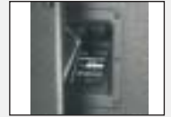
Covered input-terminal with MT-systems
